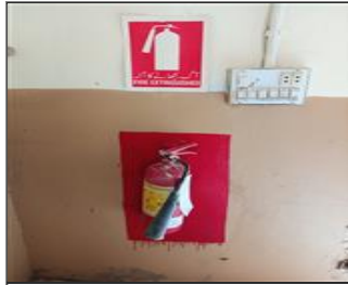
Photo of fire safety equipment Fire extinguisher.jpg
