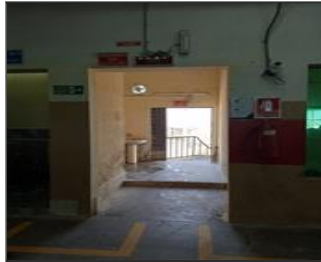
Photo of fire safety equipment Emergency exit.jpg
