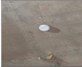
Photo of fire safety equipment Smoke detector.jpg
